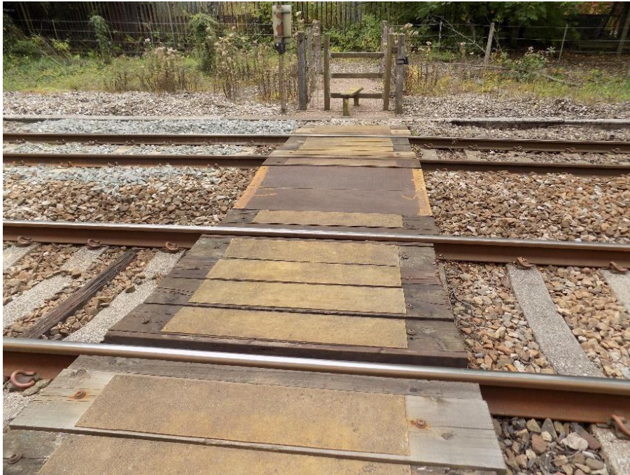
Figure 2-4.8: Level crossing deck
